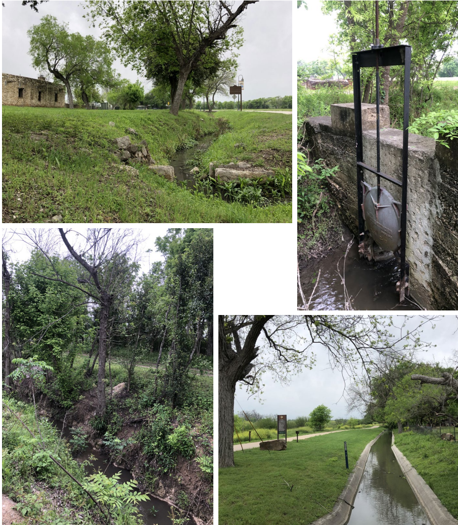
Fig. 4a – San Antonio (Texas), Remnants of a stone compuerta, or sluicagate, in a functioning acequia at mission San Francisco de la Espada (photo, 2024).
